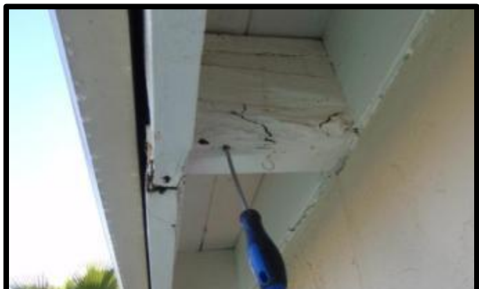
Wood rot at the back eave
