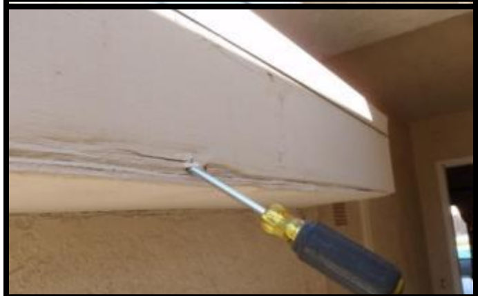
Rot at the front entry
