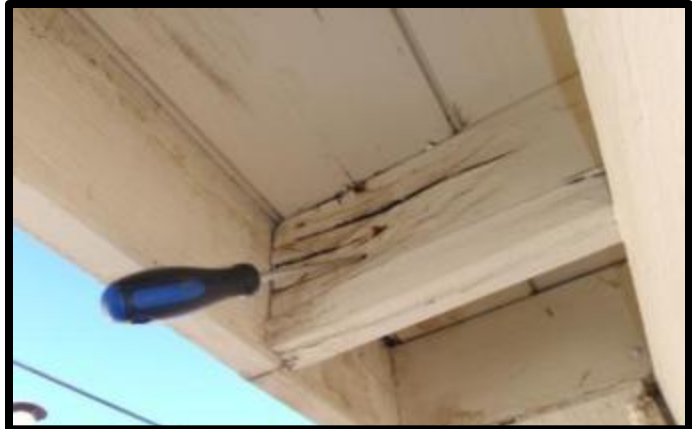
Rot at the carport
